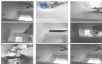
Labors and Repair Improvement of Day Care Center at Barangay San Pedro
